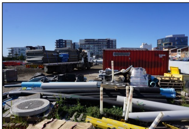
FIGURE 36: STOCKPILED CONSTRUCTION MATERIALS ACROSS SU2 (SOURCE: CURIO 2018)
